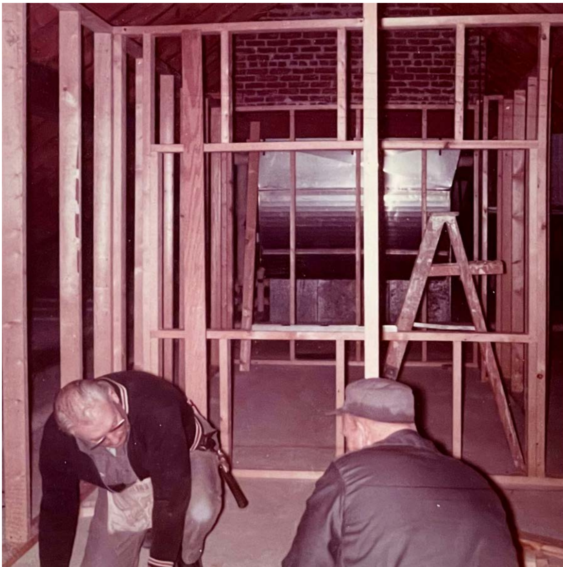
Bill Bond, head carpenter in the Facilities Department, frames the new studio in the west attic of the Memorial Building. Brickwork and HVAC in the background.
